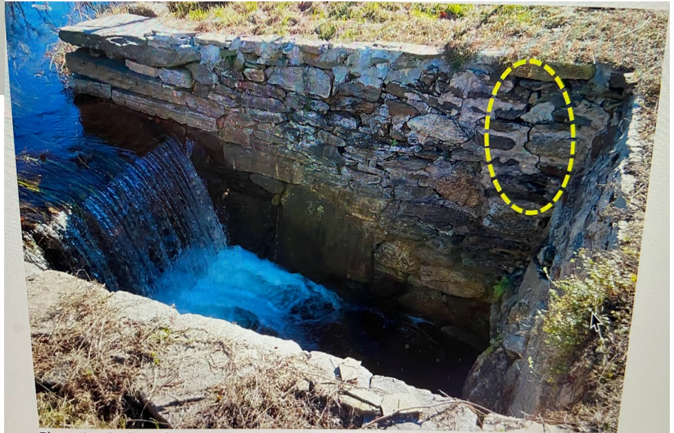
Photo 5 – The left side upstream training wall, highlighting a slightly diagonal vertical crack in the mortared masonry wall.
