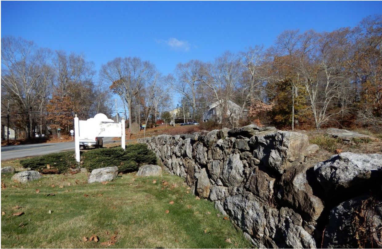
Photo 3 – A view of the right side downstream wall in stable condition, with a well maintained downstream grass area.
