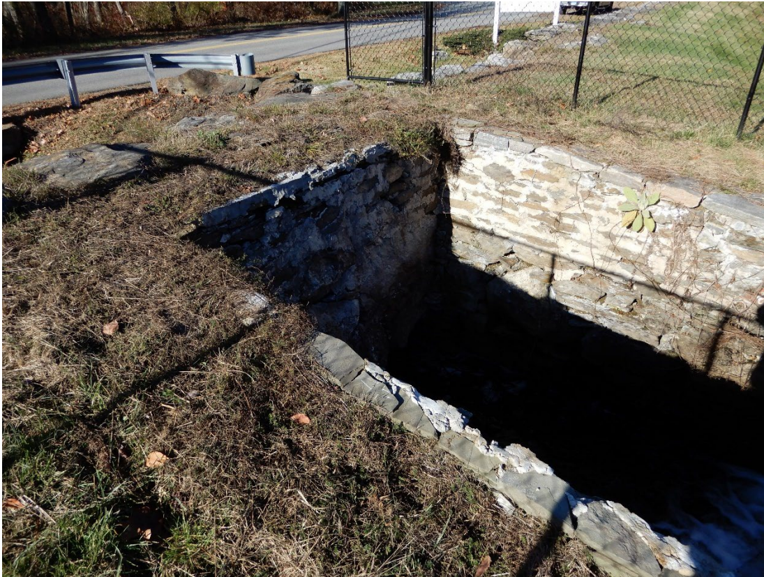
Photo 9 – The right side spillway training wall, the upper mortared section of which is in good condition.
