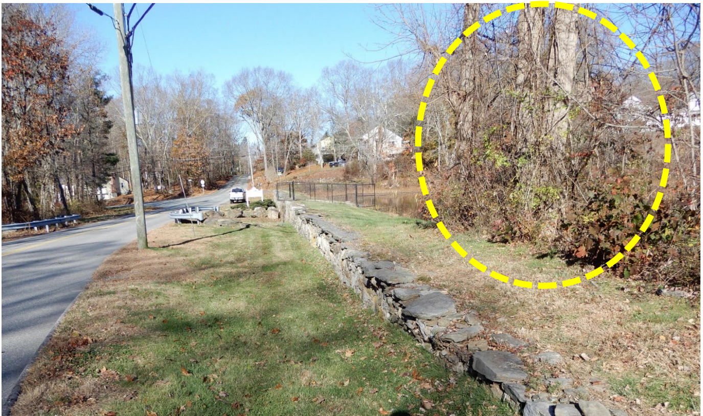
Photo 4 – The left downstream dam embankment, also in stable condition with a well maintained downstream toe area. Note, however, that there are several large trees along the upstream side of the dam, within the 25-foot limit area, which need to be removed.
