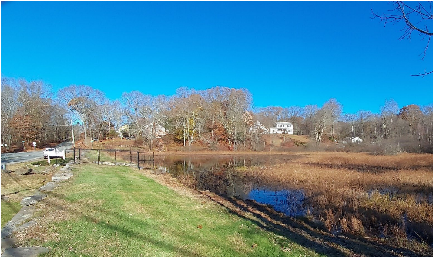
Photo 1 – An overall view of the dam from its left side abutment area. The top of the dam and grass area are well maintained.
