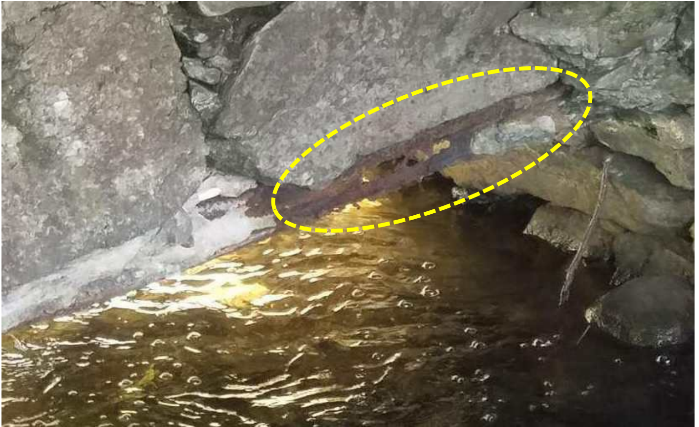
Photo 13 – A closeup of the upstream support rail showing a complete loss of the rail's web section at its right side support area. While the thickness of these sections varies and the origin of the rails is unknown, a median value should be a thickness of approximately \frac{3}{4} of an inch.
