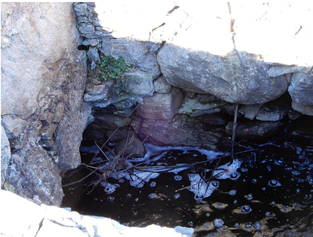
Photo 10 – The lower portion of the same right side wall section, dry stacked with void spaces and apparently missing chinking stone.
